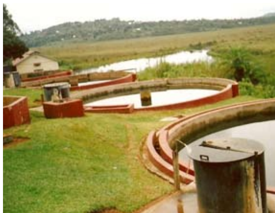
Masaka Municipal Council storage tank © UN-HABITAT
